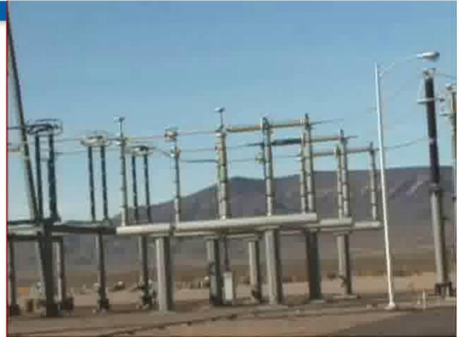
100 ft 500kV Arc on Substation Switch
